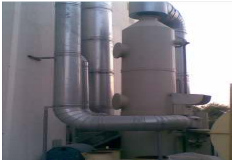
Fume Scrubbing System
