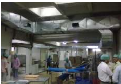
Air Cooling System
