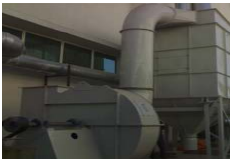
Dust Collection System
